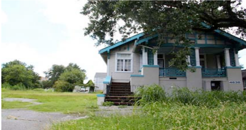
Current photo of a portion of Planned Parenthood (PP) property with dilapidated building that will have to be demolished.
